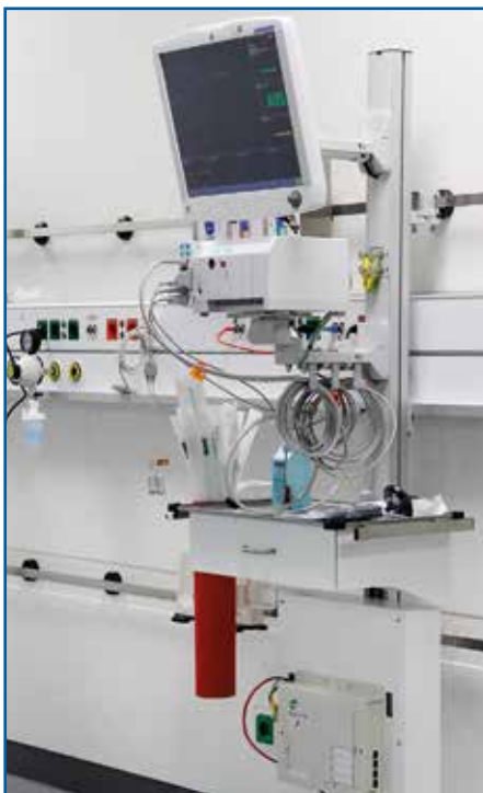
Fixing to wall supply duct and standard runner at the intensive-care station
